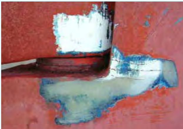
Cracking across the rudder neck close to the stock
