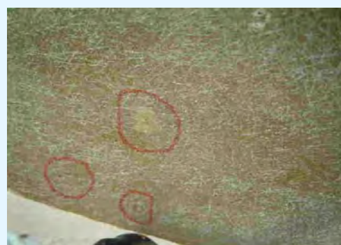
Voids beneath sandblasting easily seen
