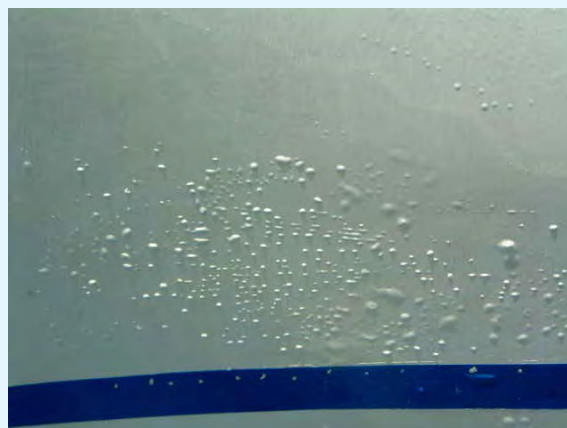
This is merely water beneath paint on resprayed GRP topsides, annoying but not a structural deterioration
