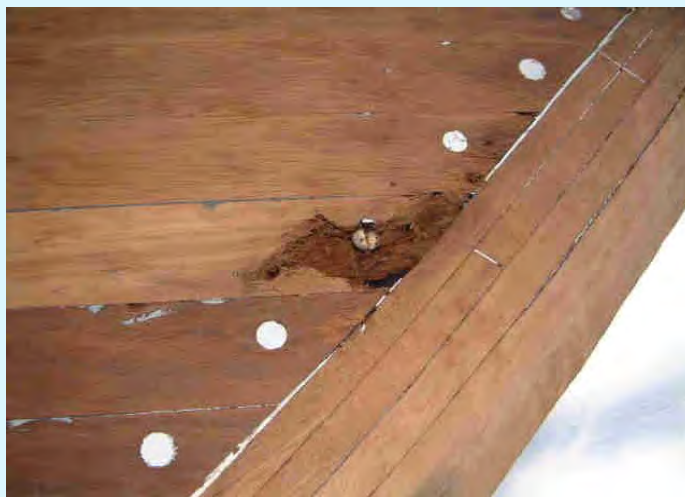
Note the narrow strips and laminated stem. Note the decay in one hood end
