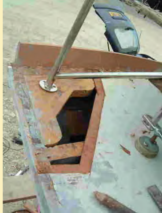
Here can be seen a series of discovering the rot, replacing all the underlying quarter knee that had completely disintegrated and the final finishing. This was caused by water leaking in the pushpit fastenings
