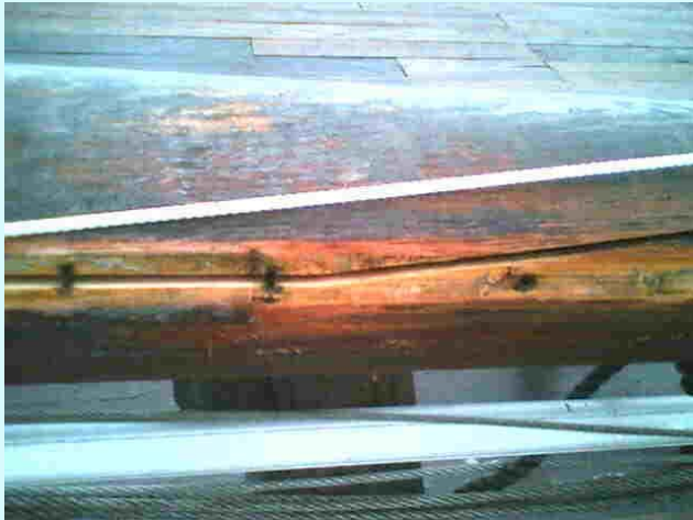
Here can be seen major glue line failure on a scarf joint extending onto the side section of boom
