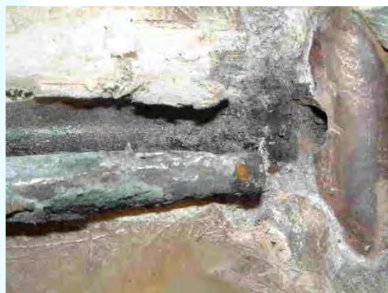
Close up of original corroded mild steel tang just push fit into bronze stock drilling
