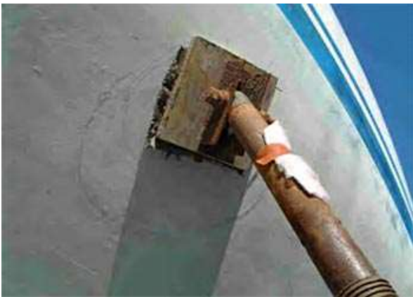
2 Stress cracks emanating from a baseplate mounting
