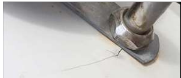
1 Stress cracks emanating from a baseplate mounting
