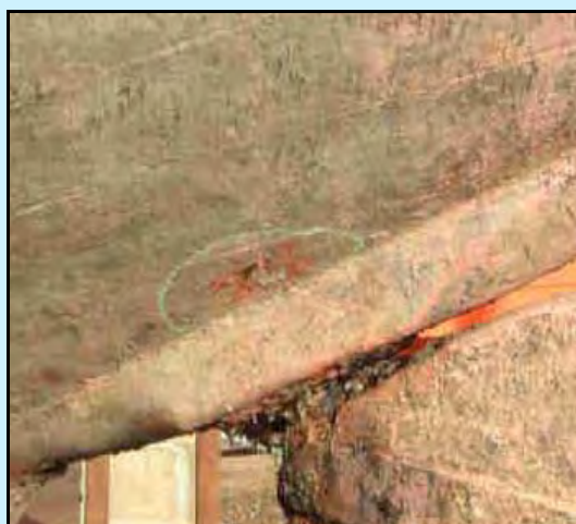
Early electrochemical damage caused by Copper Fastening contacting steel rudder tube & creating electric cell with softening to the plank hood end
